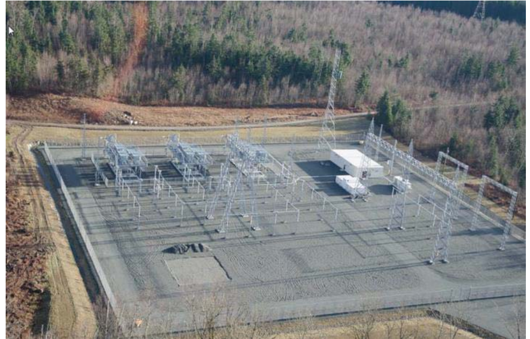
Example of a Capacitor Station.
