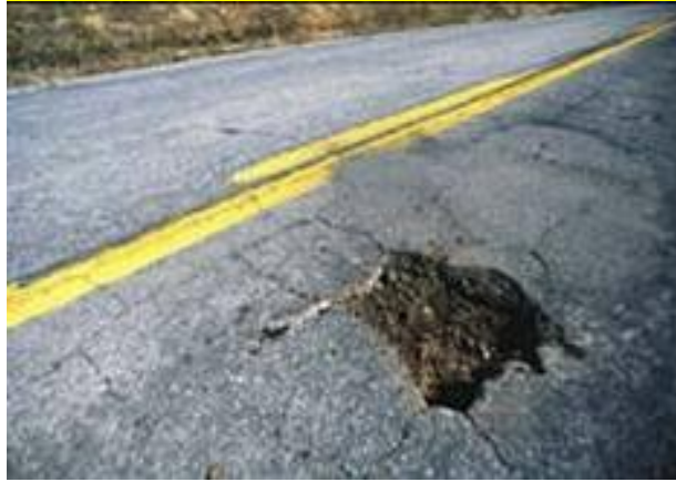
Figure 6. Potholes are a common issue on Prince George roads. (Photo: courtesy of City of Prince George)
