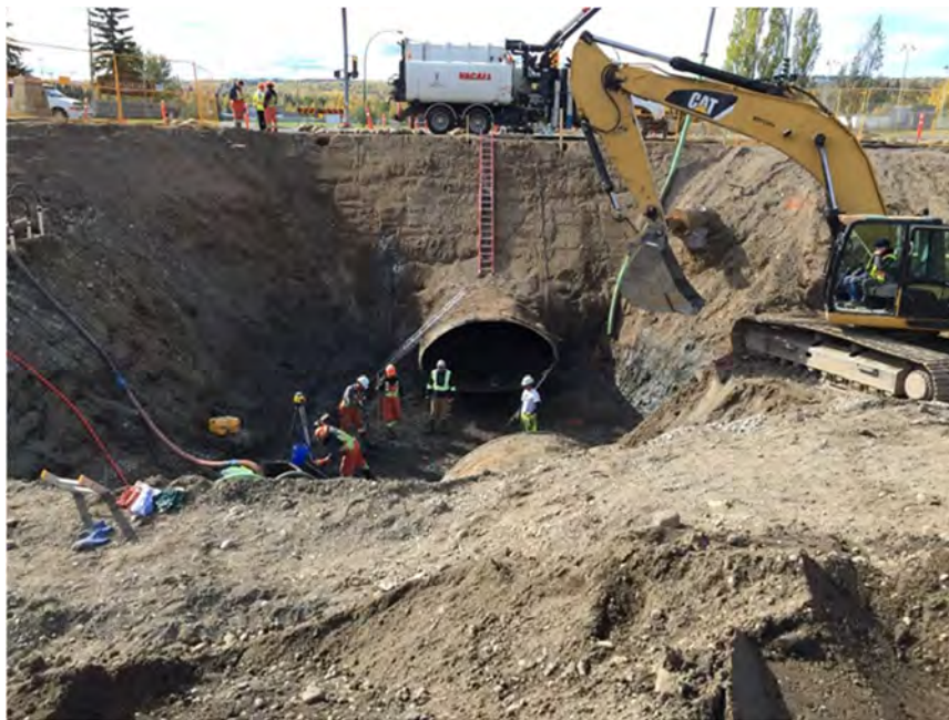
Figure 5: Winnipeg St. Sinkhole (2018) - $1.7M
