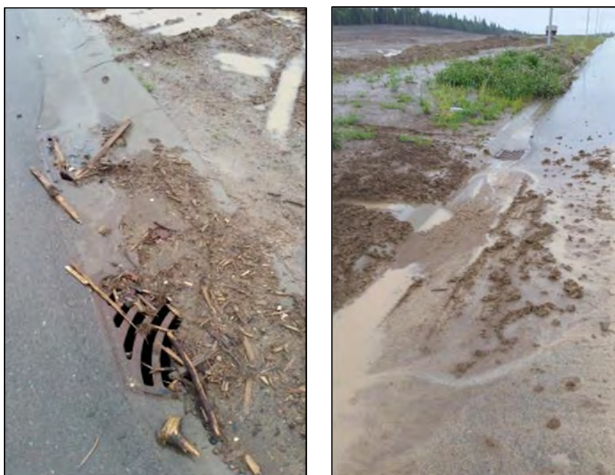
Figure 6: Erosion and Sediment
