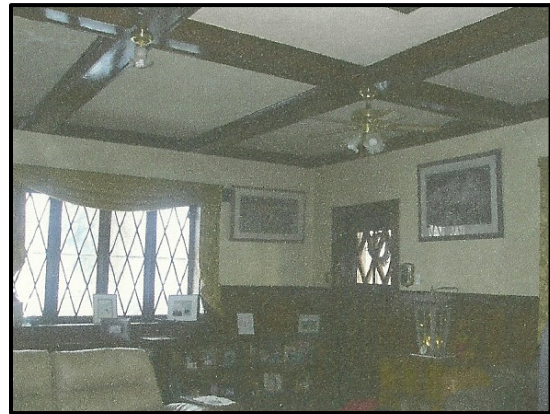
Photo 2: Coffered ceilings on main floor, wallpaper finishes, wood wainscot. Diamond-shaped windows with wood muntins
